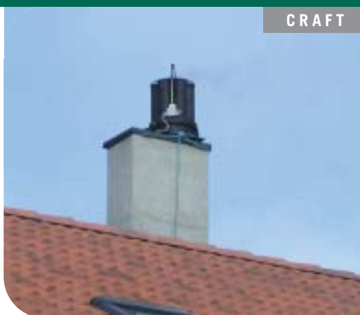
CleanAir unit mounted on a chimney top. © APP
